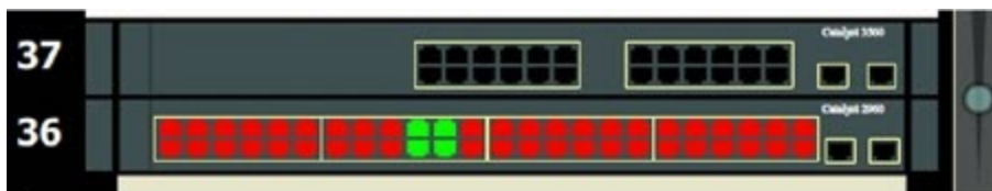
Figure 223 Deployed switch showing red and green port status icons
